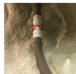
TUBI G TUNNEL G TUNNEL HOSES
